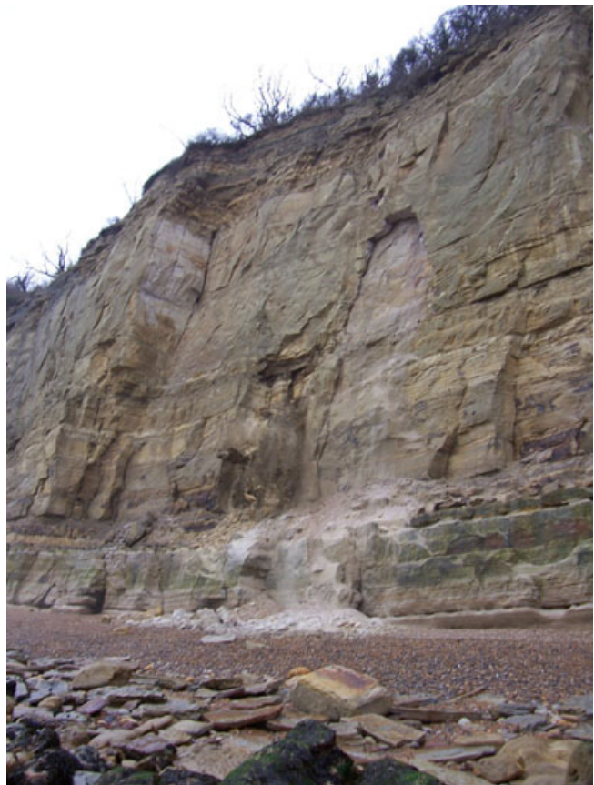
Figure 2: Start of the collapse with material caught in 'free-fall'
